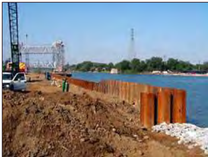
AlliedSignal, a former steel mill site, is the future home of a new automotive supply manufacturing campus in Chicago. The seawall was installed to stabilize the ground along the Calumet River.
