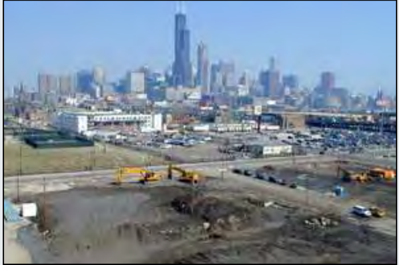
Remediation work south of 14th Place (Winter 2001) Graphic courtesy of the South Campus Development Team, LLC
