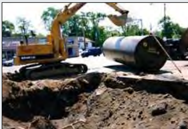
Removing an Underground Storage Tank (Photo Courtesy of Delta Environmental Consultants, Inc.)
